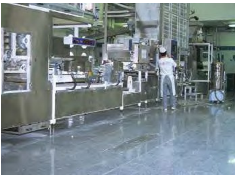
Type SBVE in use in a food processing plant
